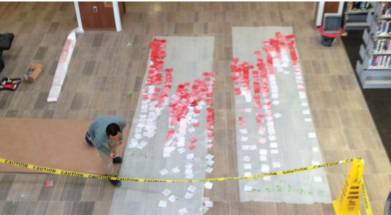
The strands were organized prior to arriving at the site to maximize efficiency.
