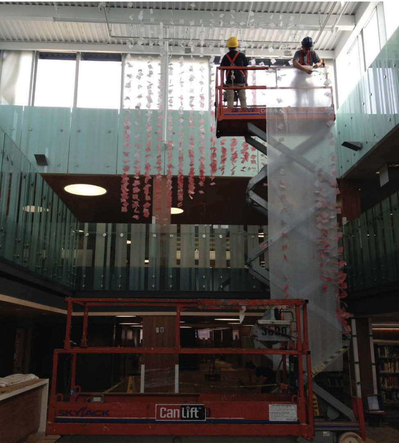
Each rise of the scissor lift installed a full row of 18 strands.
