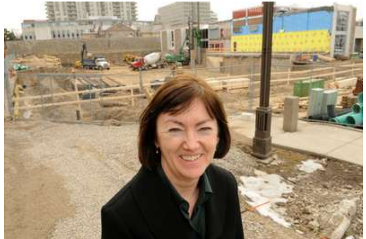
Library expansion Chief executive officer Sonia Lewis stands near the construction at the back of the Kitchener Public Library. Philip Walker/Record staff
